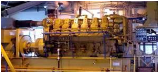
Figure 6: Generator of the Kosrae Utilities Authority. (Source: DoI, 2006)
