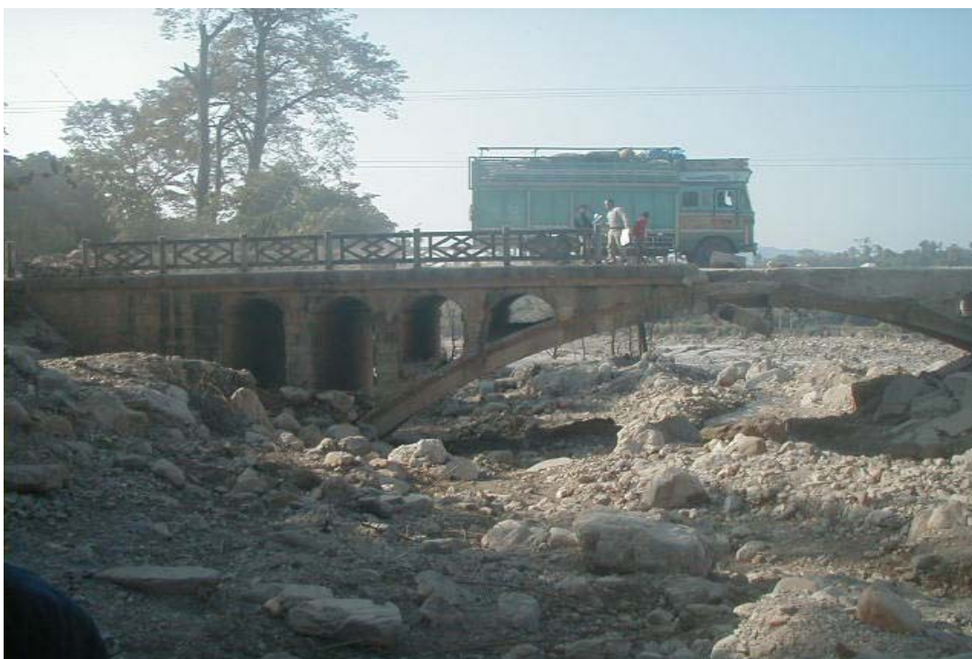
Plate 4: Damaged Bridge in the Khahare Khola, Mugling Narayanghat Road section.
