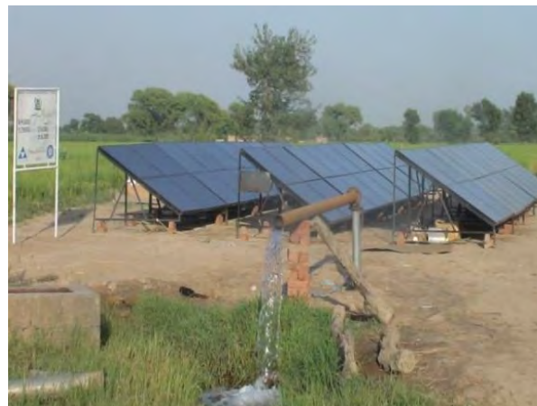
Solar powered irrigation system at Nankana Sahib, Punjab
