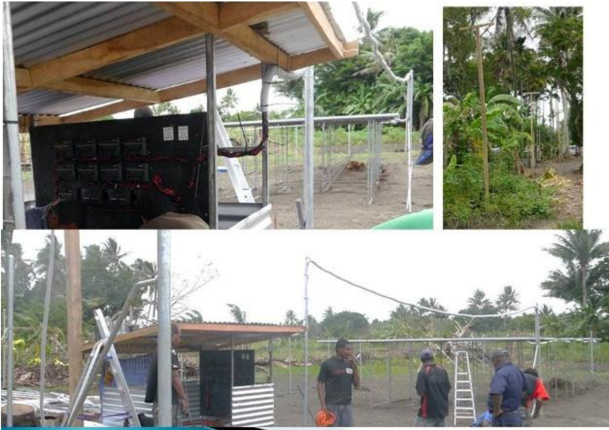
Community-based Solar Farm panels in the Aroma Coast, Central Province
